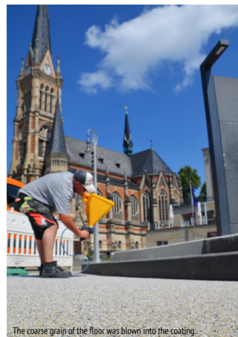
The coarse grain of the floor was blown into the coating.
